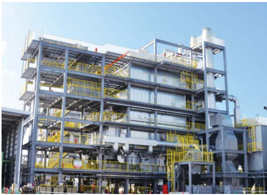
Biomass boiler in the Okayama Plant
